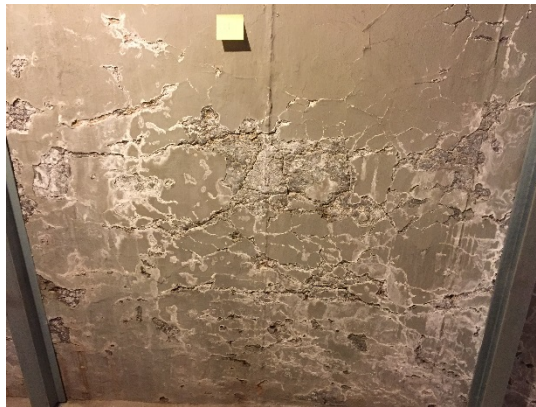
(c) map cracking
