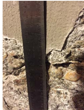
d) crack opening (>4mm)
