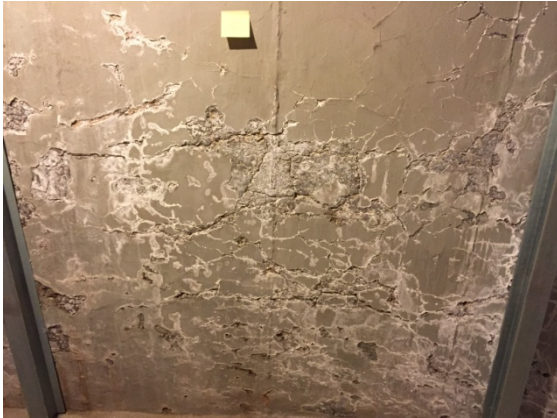
a) map cracking
