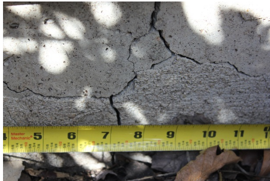
(c) wide crack opening
