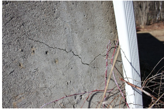
(c) map cracking
