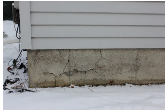
(c) map cracking
